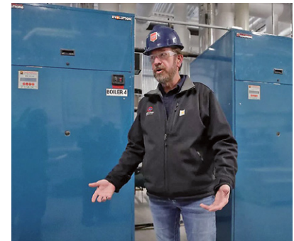
Masters Gallery Foods, Oostburg, incorporated geothermal heating and other technology to increase sustainability efforts
